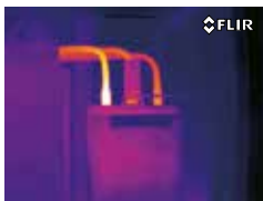
Poor connection and internal damage
