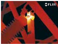
Incorrectly secured connection
