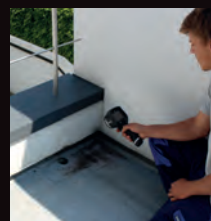
Discover leaks in roofs
